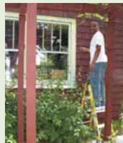
A fresh coat of paint is one result of a board work day in May.
